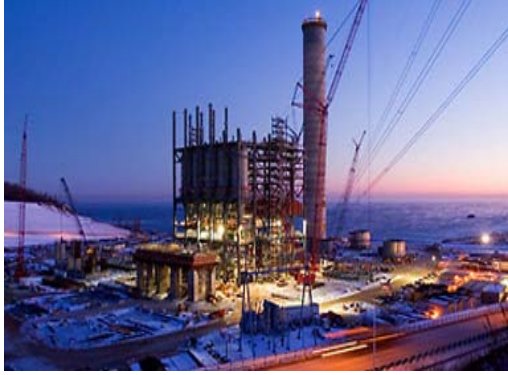
Oak Creek Power Plant; Milwaukee Client: Bechtel
